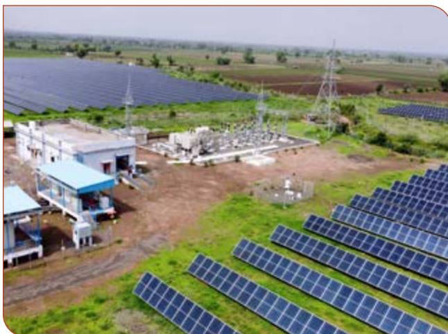
Solar Power Plant
