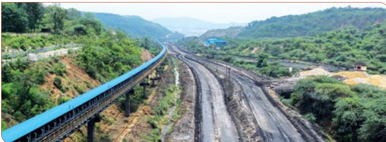
RCML - Inpit Conveying System & Coal Handling Plant
