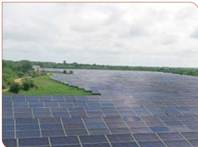
Solar Power Plant, Achampet, Telangana
